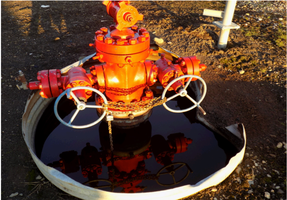
Figure 2: Leaks which cause human harm and environmental damage are a routine part of fossil fuel extraction
